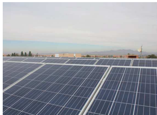
Solar panel plant on the rooftop of the hospital building
