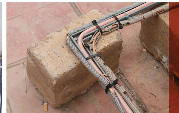
Wires on the solar panel plant corroded due to extreme heat
